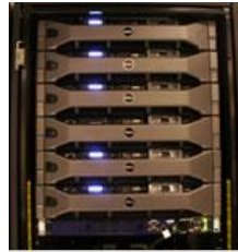
Dell™ PowerEdge™ R815 11-node cluster
